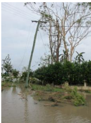
Flooding in Ingham
